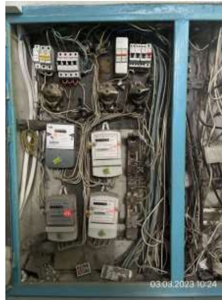
Actual condition of the floor metering panel in an apartment building
